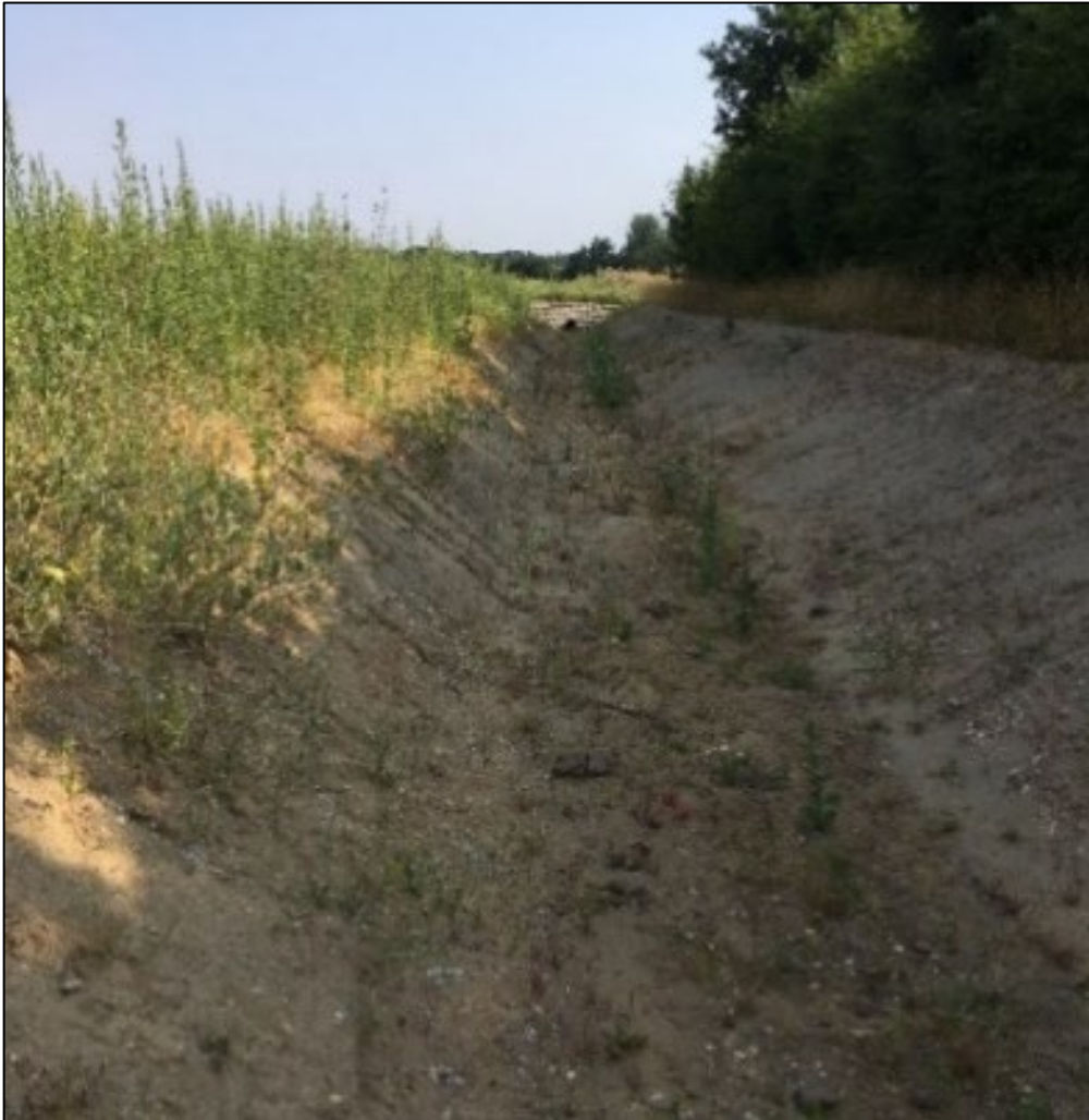
Photo 10: Photo showing a newly created channel as an extension of a watercourse, North Norwich, Norfolk (image E Simpson @ NCC LLFA).
